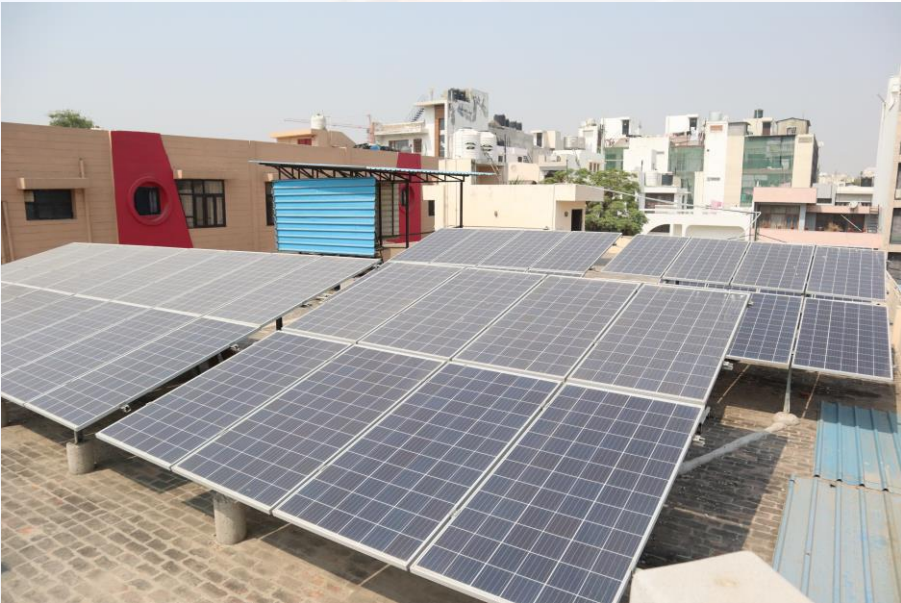
15 KW rooftop solar system in Karkardooma, Delhi
